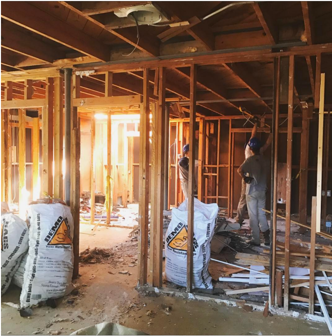
Craig Hatch and other employees at E2 Creative work together to remodel a coffee shop. (Photo by Sam Landess)
